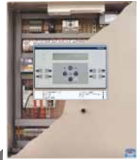
THE ELECTRICAL CONTROL PANEL
